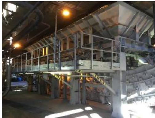
Gambar 36. Ash Handling Unit (Sumber: LGM Industries)
