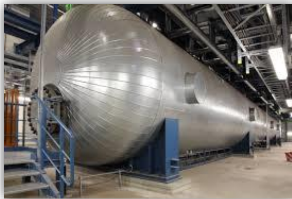
Gambar 25. Boiler (Sumber: General Electric)
